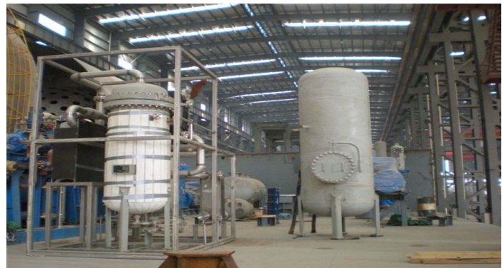
Vessel compressor unit is being assembled at the workshop of Shenghui Gas Chemical Systems, in which aims at being an advanced Cargo System provider not only a Cargo Tank fabricator.
